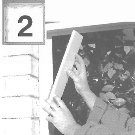
2 Place the Ezylay expansion material in both verticals of the Ezylay frame ensuring it extends from top to bottom.
